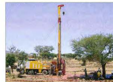
Above: a job site in Ethiopia with rig model M.I.28 at the moment the crew strikes water
