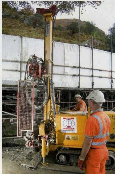
The purpose of the project was to stabilise the conduit section of the Thirlmere Aqueduct at Nab Scar
