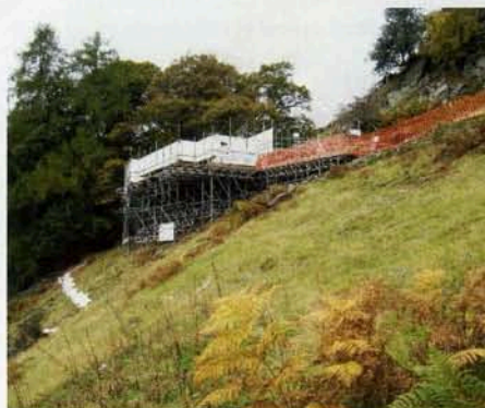
Bachy Soletanche working on a 440m fell in Nab Scar, Lake District, to conduct remedial works on the United Utilities-owned Thirlmere Aqueduct
