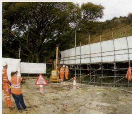
A platform off a 40° cliff face had to be installed to enable remedial works to proceed
